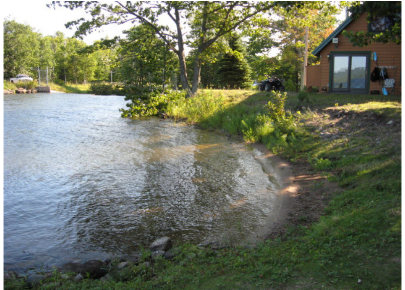
Erosion of the shoreline is clearly visible in the bank along the right side of this photograph. The dam is seen on the upper left-hand corner of the photo.
