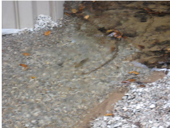
Adult spawning salmon are seen moving upstream through the diversionary channel all the while the box culvert is being installed.
