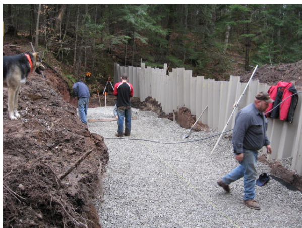
New bedding material was installed in preparation for the new concrete box culvert.
