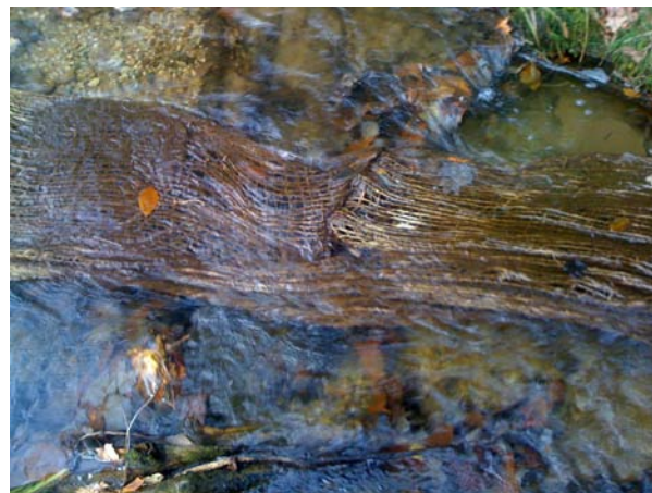
Jute matting was installed downstream from the Floc Logs and the construction site. This collection field captured the flocculated particles from reaction of the Floc Logs and sediment.
