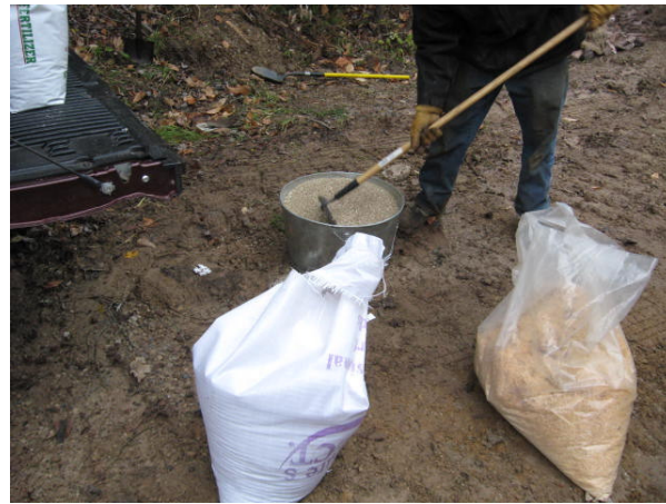
Polymer powder, fertilizer and seed were mixed together to be used to start the stabilization process on the all the bare disturbed soil along the edges of the road, ditches and all the places water will flow to the stream.
