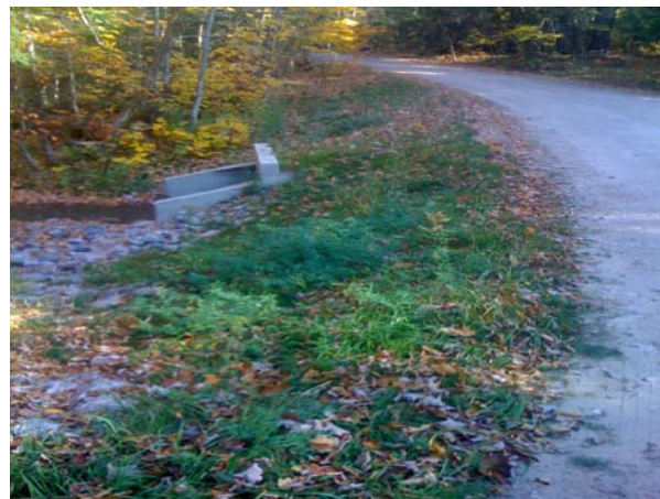
The road stabilization is complete and vegetation is established. The above photos were taken one year after the completion of the project.
