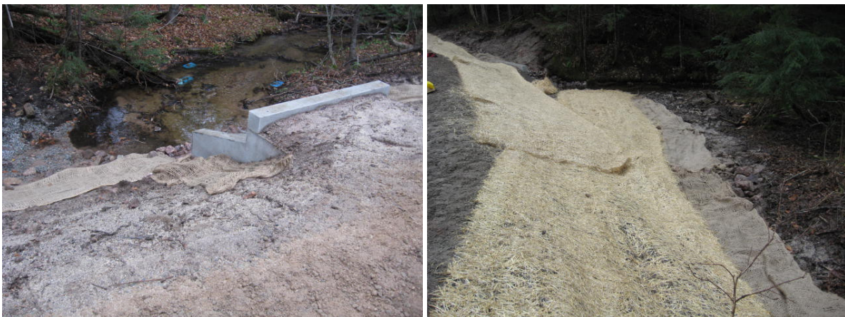
Polymer enhanced straw matting and jute was installed everywhere on the site except the road surface.
