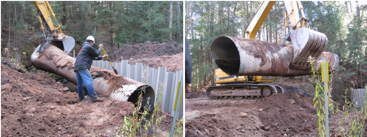
With all of the water diverted, the old culvert could now be removed.
