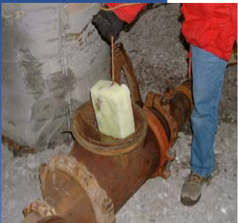
Floc Log placement within tee cage
