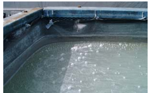
Clogged geotextile filter of initial system
