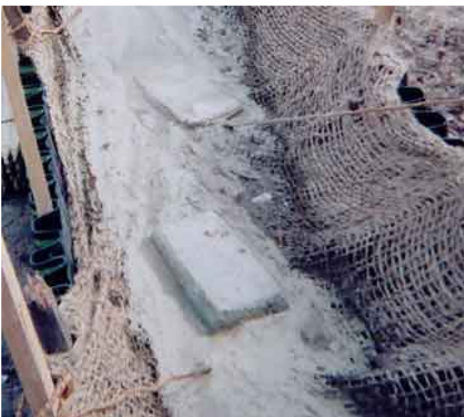
Reaction of the turbid water with the Floc Logs® caused the sediment to bind together and collect on the jute matting.
