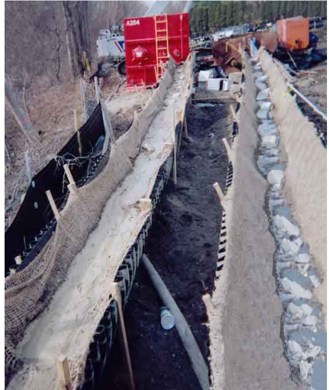
The Floc Logs were only placed in the first 50 feet of the split pipe system; rocks were placed in the system further down to assist with mixing and slow the velocity of the water.
